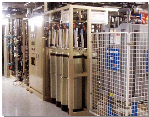
Water Treatment system using Liqui-Cel® Contactors at Tohoku University
